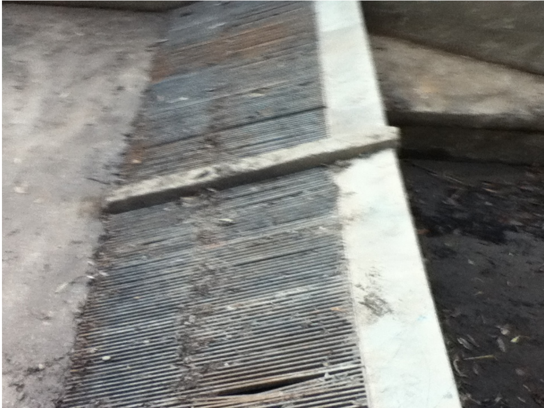
Figure 2.9: the surface gross pollutant trap at Lime Kiln Bay.
