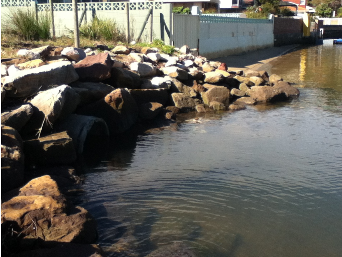
Figure 2.1: The stormwater release pipes at Kyle Bay
